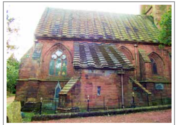
North facade of the old church. Looking a bit shabby prior to present work.
